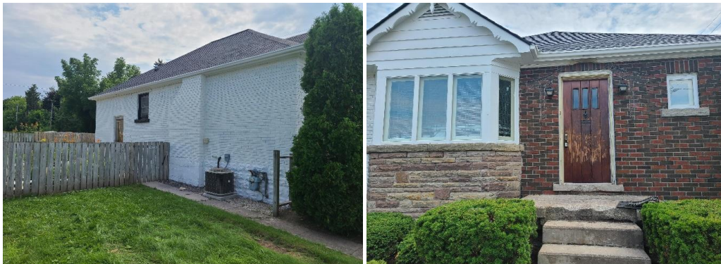
Figure 3 Subject property on July 23, 2021. East facade painted, chimney and entrance roof removed. Majority of front and west facades remain unpainted (By-law Enforcement Photos)
